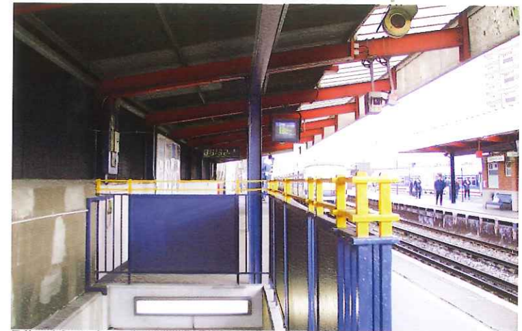
Dilapidated and out dated railway station platforms
