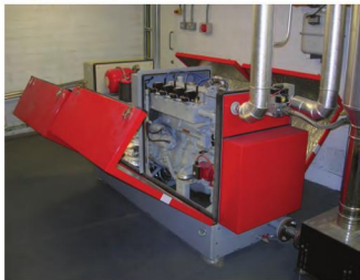
11.13 On-site power generation with CHP engine.
